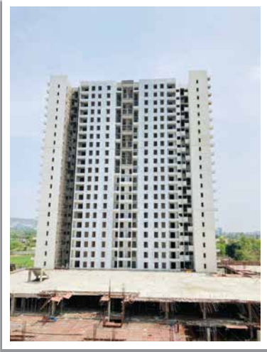
Y1H-B- Kitchen otta fixing work is in progress on 19th floor, wooden door frame fixing work is in progress 16th floor
