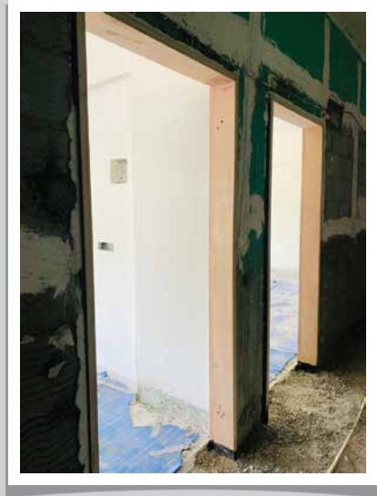
RYAN SCHOOL- Door frame fixing work is in progress on 1st floor
