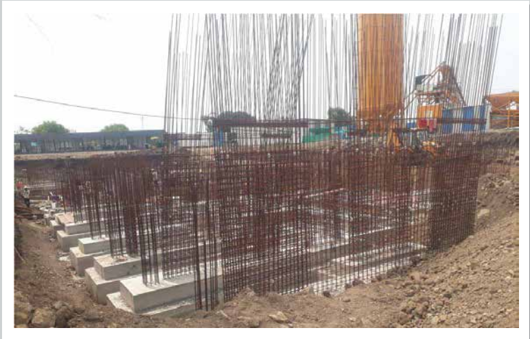
Y1In-C1C2- Footing casting work is in progress, backfilling work is in progress
