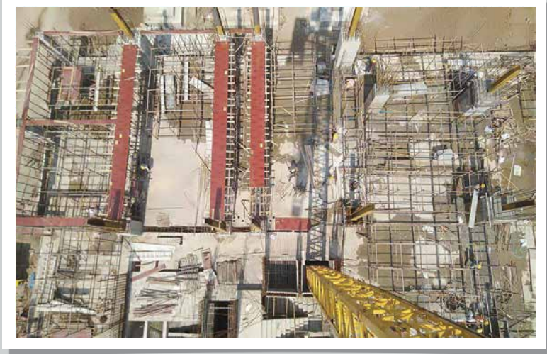
VJ GRAND CENTRAL- Ground floor slab (part1) beam bottom work & shuttering work is in progress
