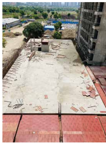
Y1H-MULTI PURPOSE HALL- Shuttering work for LMR & parapet wall is in progress
