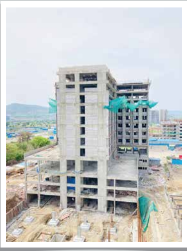
VJ ONE AVENUE- Basement raft casting work is in progress, blockwork is in progress on 6th floor
