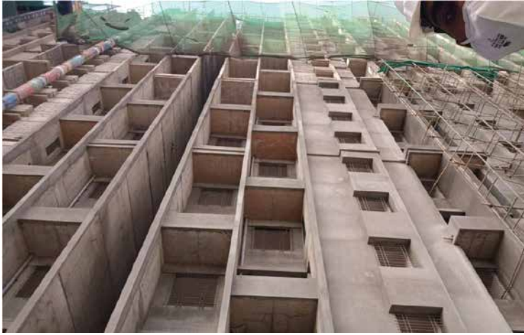
Y1WC-B- 23rd floor slab (terrace floor) casting work has been completed, above terrace OHWT shearwall reinforcement, shuttering work is in progress
