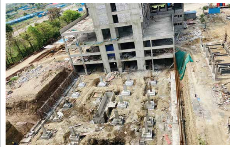
VJ ONE AVENUE- PCC & Footing work is in progress, Water tank PCC work is in progress
