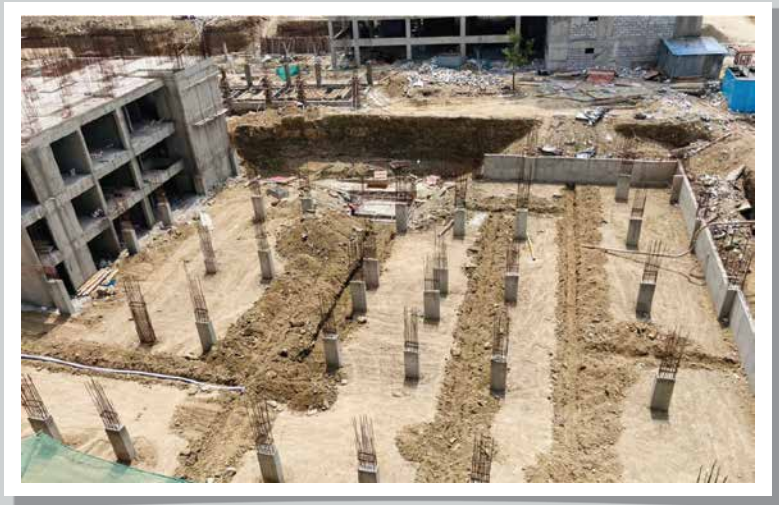
Y1H-PODIUM PH-2-(block D) - Column & retaining wall work is in progress, UG services work is in progress
