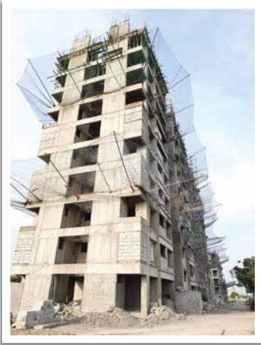
YSNW-A- Shearwall work is in progress on 11th floor, blockwork has been completed till 5th floor, gypsum plaster work is in progress on 2nd floor
