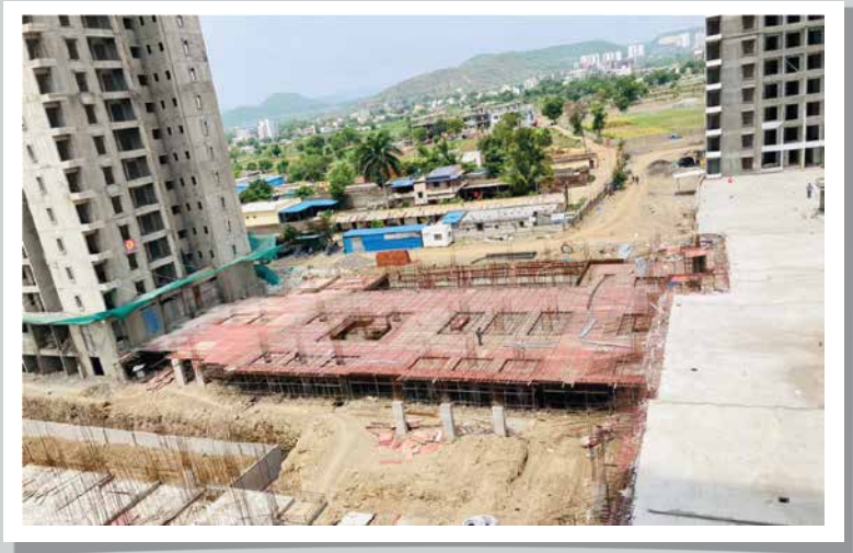
Y1H-PODIUM PH-2(block C)- Tendon laying work is in progress for 1st slab
