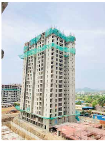
Y1H-E- Steel fixing & shuttering work is in progress on 21st floor, blockwork is in progress on 16th floor, waterproofing work is in progress on 8th floor
