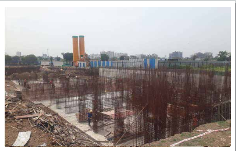
Y1In-D1D2- Basement raft reinforcement and casting work is in progress, 1st slab shearwall shuttering & reinforcement work is in progress
