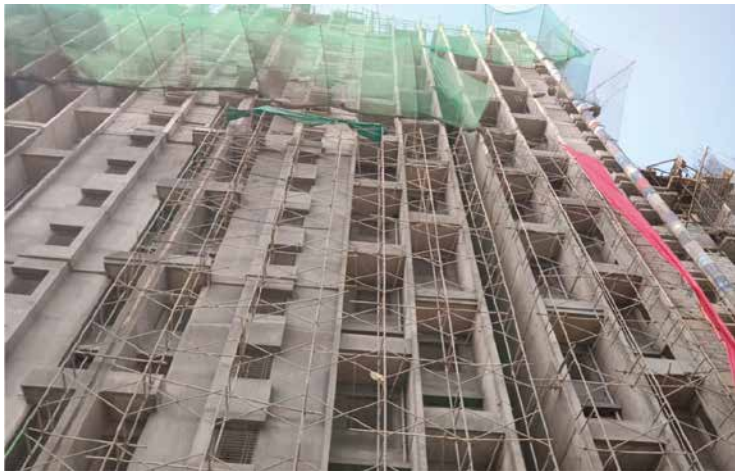
Y1WC-C- 23rd floor slab (terrace floor) casting work has been completed, above terrace OHWT shearwall reinforcement, shuttering work is in progress
