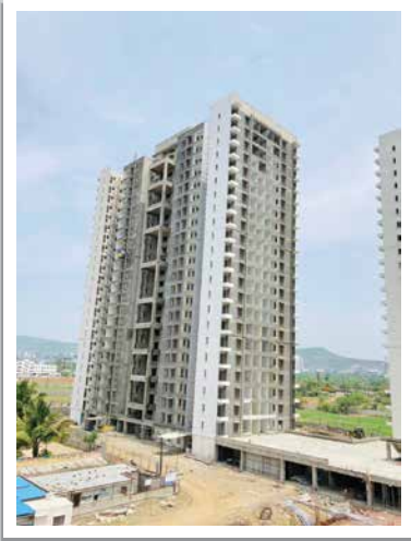
Y1H-A- Kitchen otta fixing work is in progress on 19th floor, wooden door frame fixing work is in progress 18th floor
