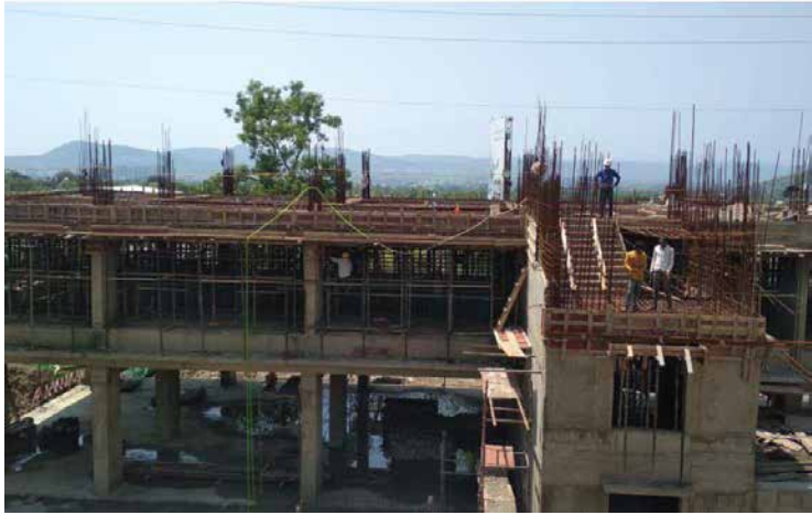
VJ HAPPINESS STREET- 2nd floor slab has been completed, 3rd floor slab shuttering work is in progress
