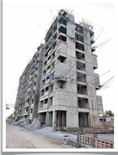
YSNW-B- 10th slab shuttering work is in progress, blockwork is in progress on 6th floor, gypsum plaster work is in progress on 3rd floor
