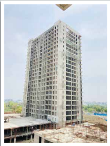
Y1H-C- Blockwork has been completed till 21st floor, gypsum plaster work is in progress on 17th floor, waterproofing work is in progress on 8th floor
