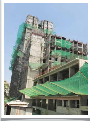
Y1WC-D- 13th floor slab casting has been completed, shearwall reinforcement, shuttering & casting work is in progress
