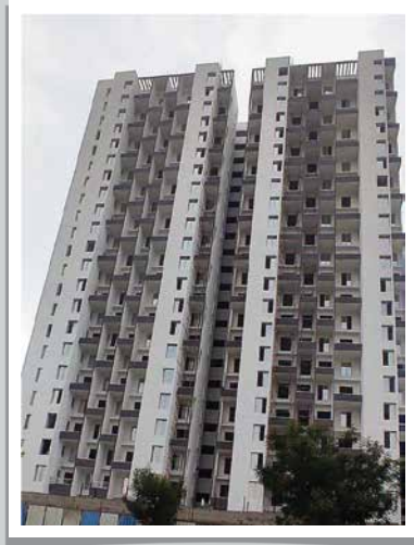
YE-A2- External painting final coat work is in progress, south side flats aluminium windows fixing work is in progress
